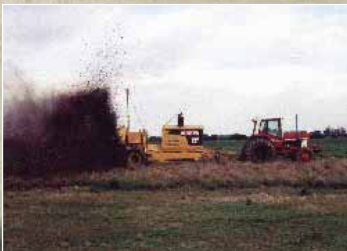
Rotary drainer in action.
